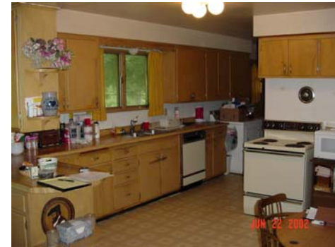
BEFORE: The cabinetry and finishes were outdated.
